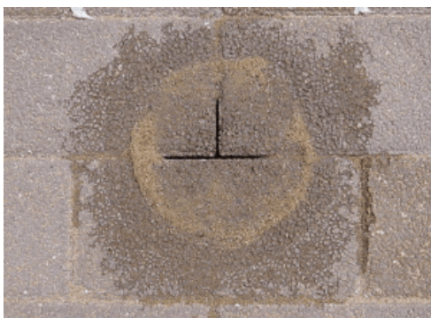
Photo 2. Loss of joint sand in permeability test.
